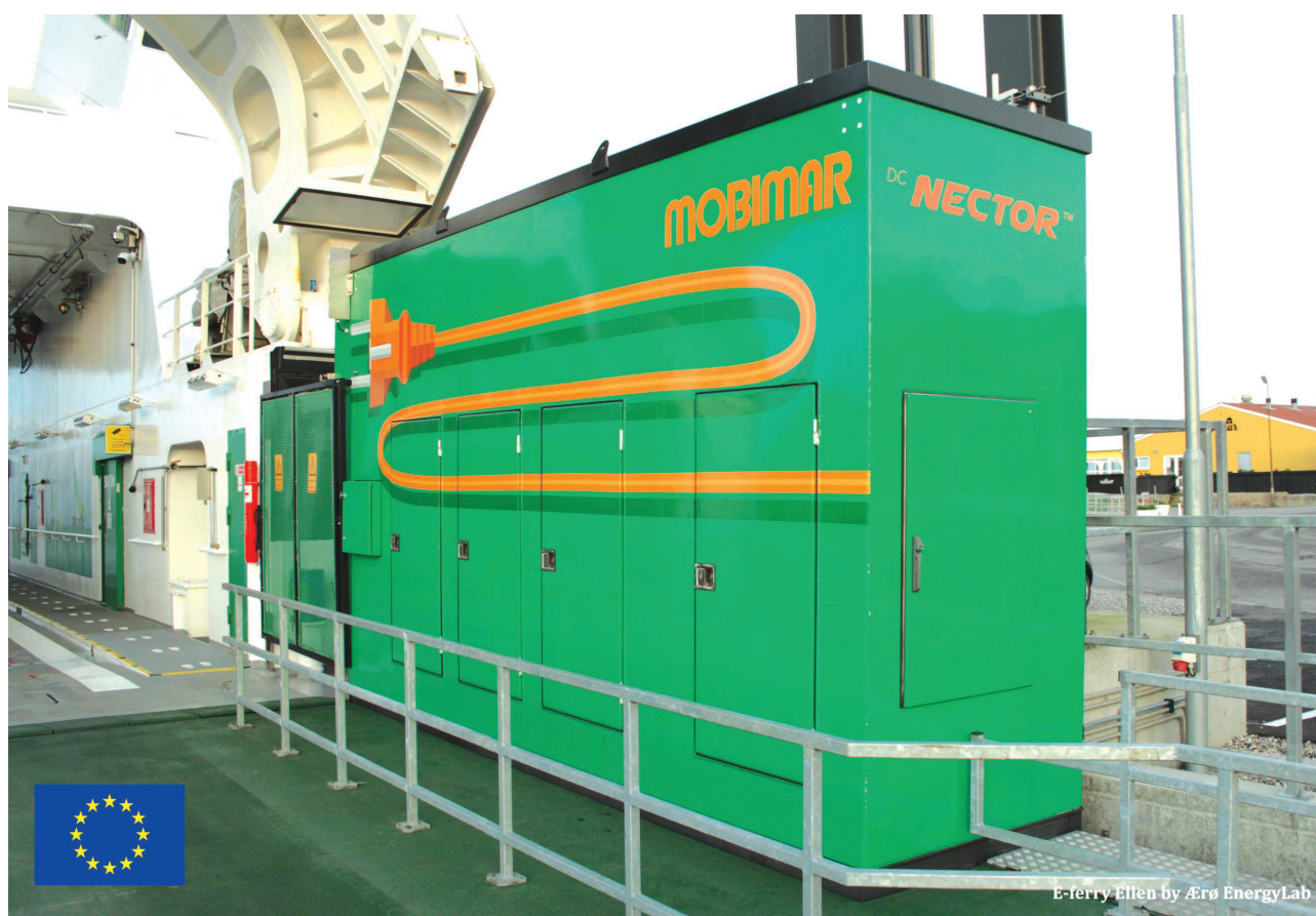
Image A5.7 Electrically powered ferry for passengers and vehicles
