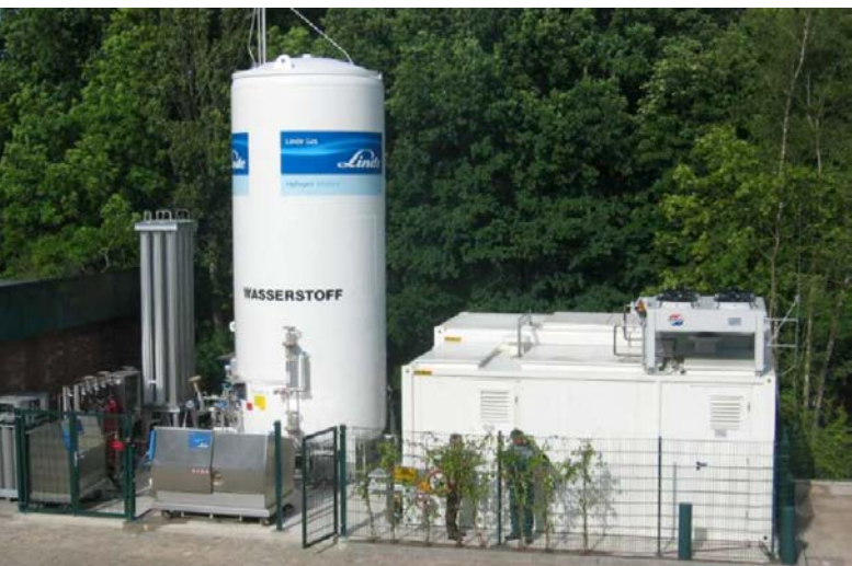
Figure A.15: H2 compression and storage station
