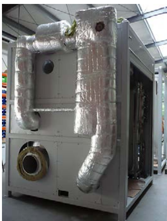
Figure A.3: The media module containing support systems for the fuel cell
