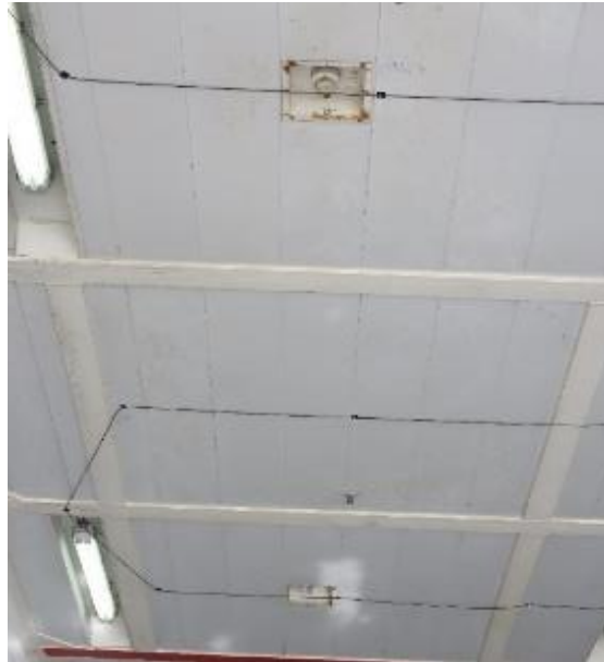
Figure 19. Position of the fibre optic cable in relation to existing conventional detectors.
