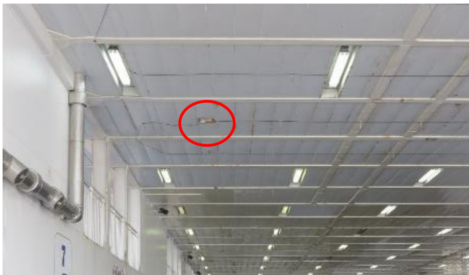
Figure 20. Existing detector (circled in red) and fibre optic cable positioned at a side opening.
