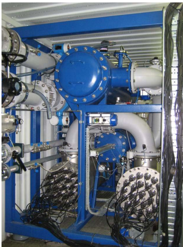
Figure 8 View inside the container with the OPS (Photo courtesy of Mahle).
