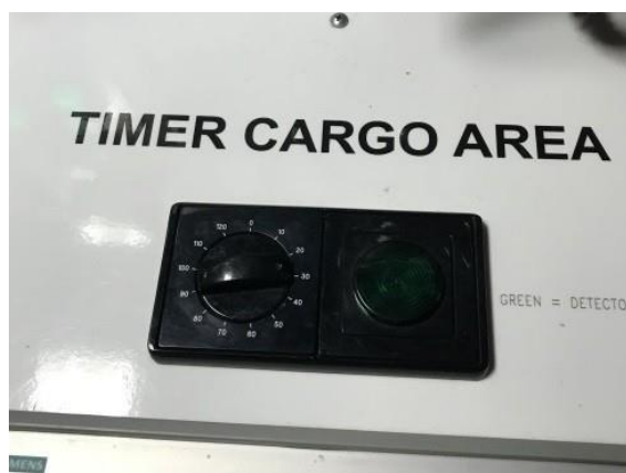
Figure 10: Timer (2 h) for inactivation and reconnection of fire detection system on (all) ro-ro spaces
