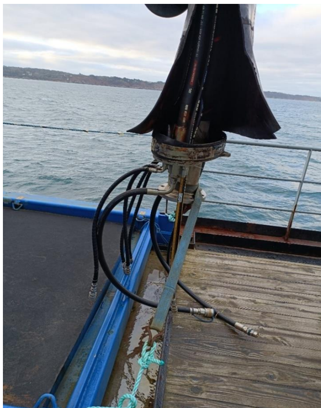
Figure 3. Umbilical hose cut for repairs inside.
